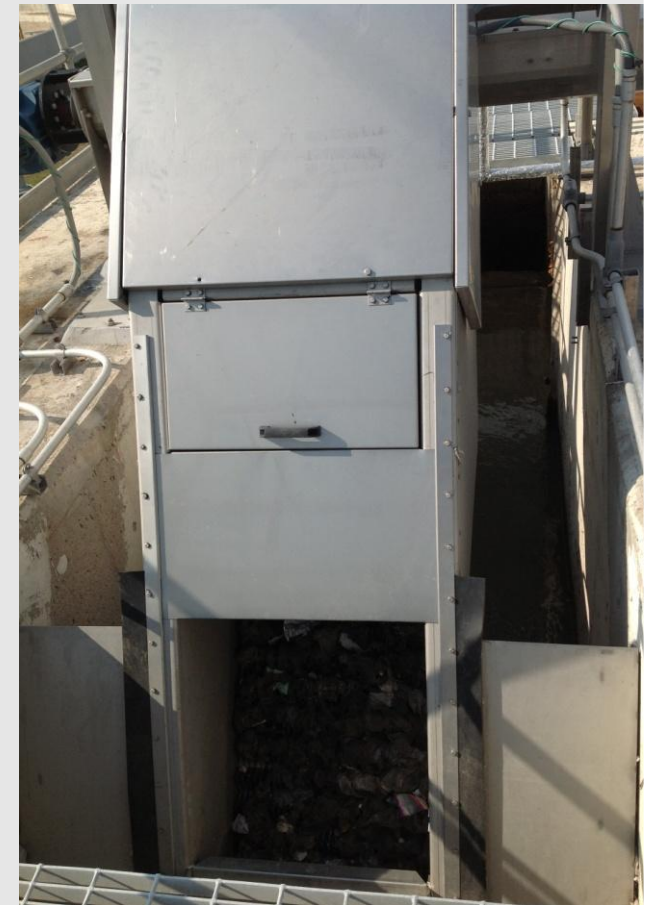
New Bar Screen and compactor
