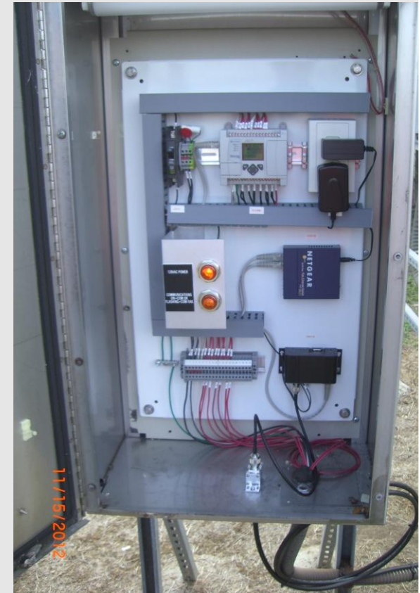
New SCADA Panel
