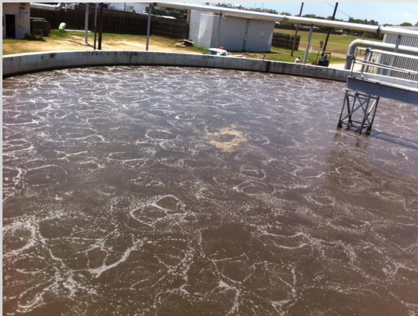
Basin with Fine Bubble Diffusers
