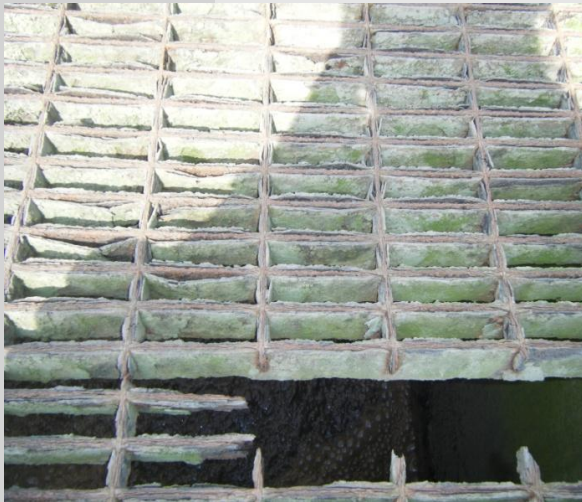
Rusted and Rotting Grates
