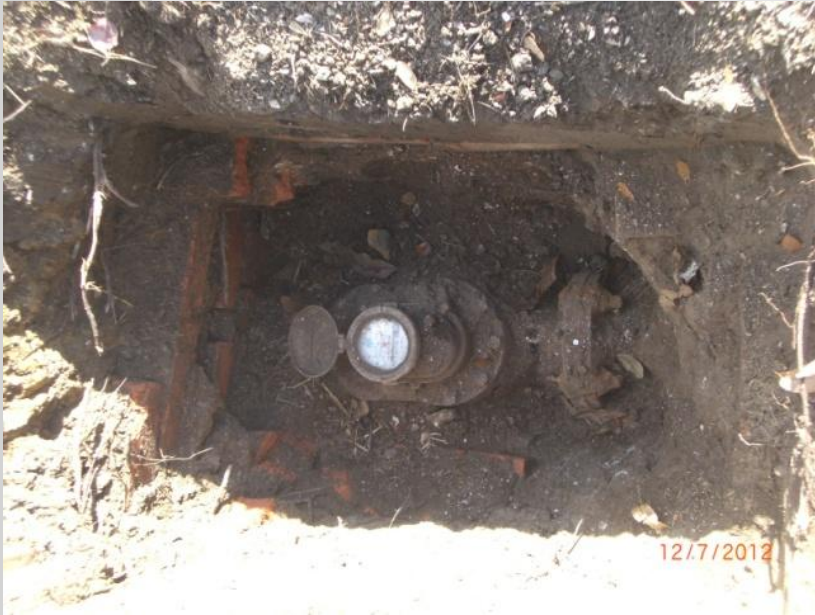
Water Meter before upgrade
