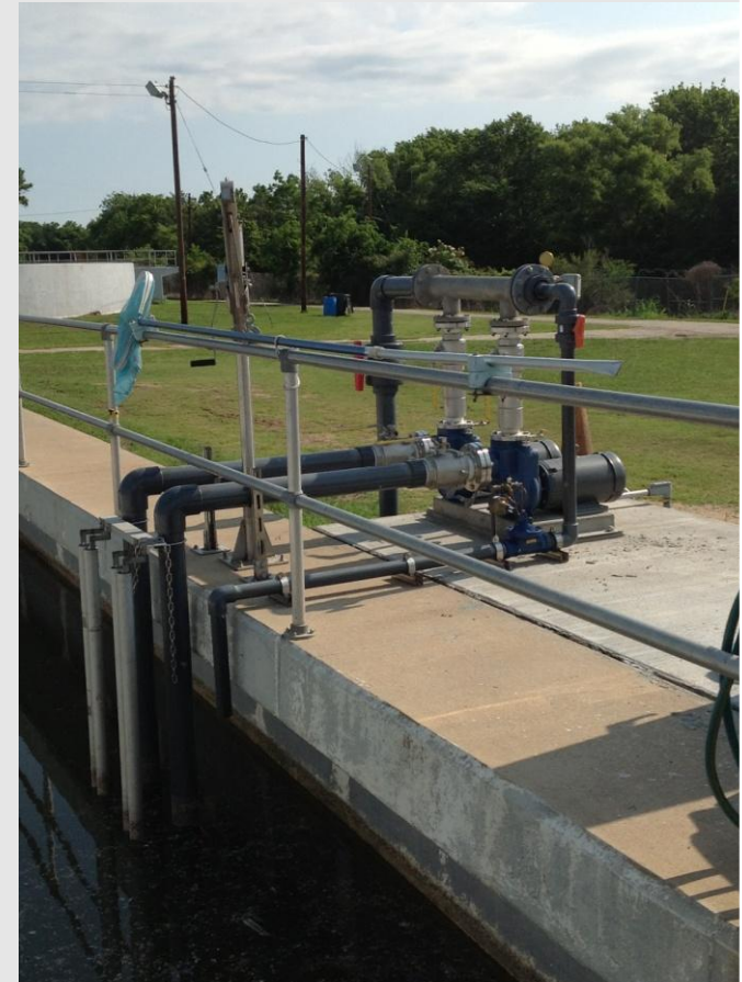
New Non Potable Water System Pumps
