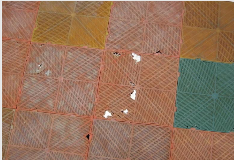
Existing Drying Beds – damaged tiles
