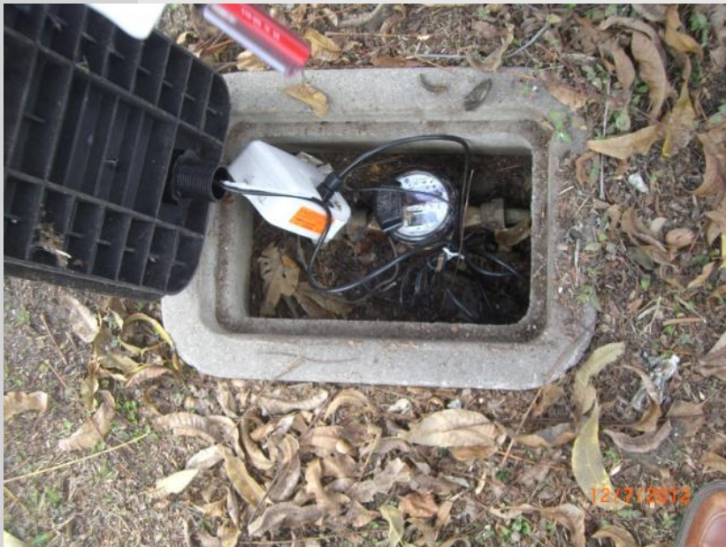
Water Meter After Upgrade
