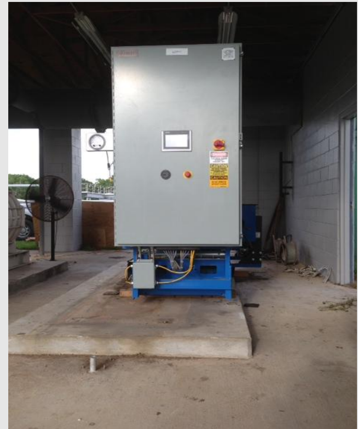
New Blower Panel
