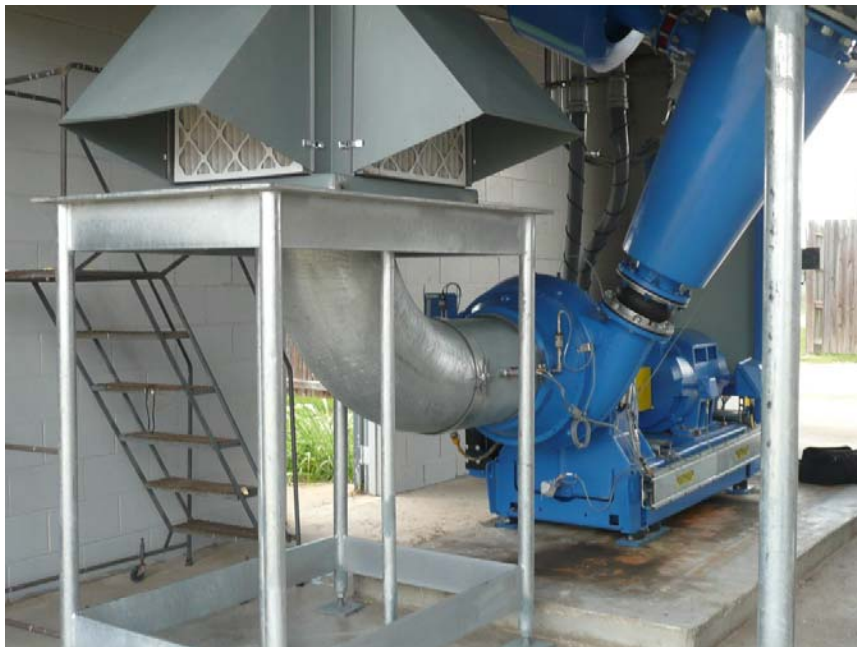
Figure 6: New 350 HP Siemens Turblex Blower (Alternate View)
