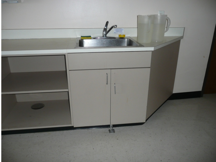
Figure 32: New Pedal Valve Controls on Sink (Kitchen)
