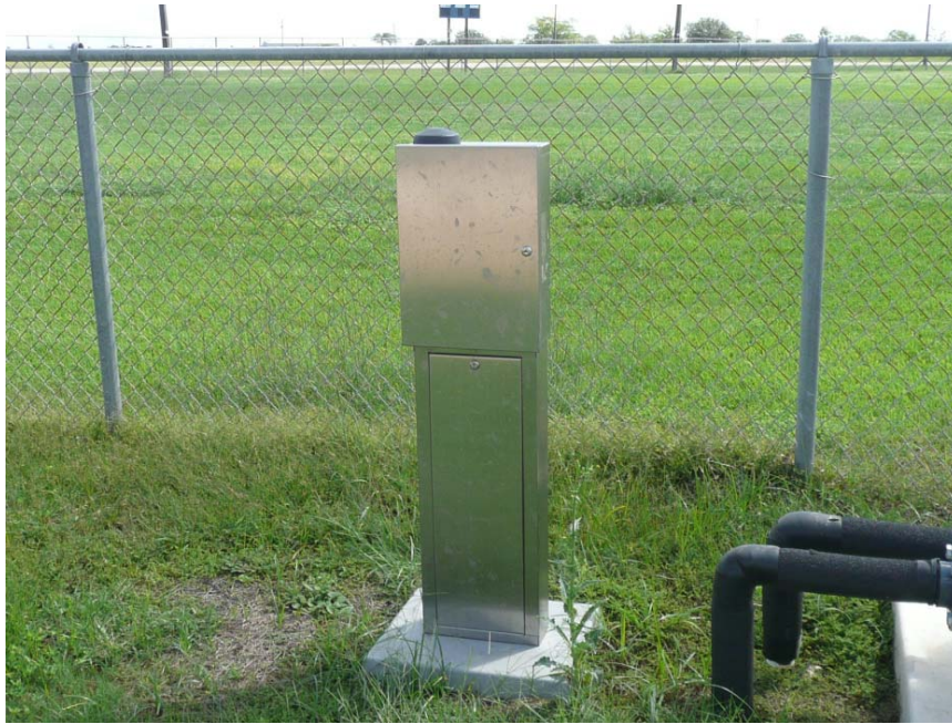
Figure 34: Rain Sensor and Flow Sensing Meter for New Controller
