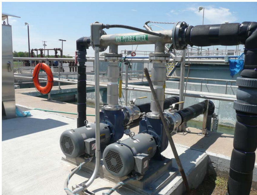
Figure 13: Two New 15 HP Non-Potable Water Pumps with VFDs
