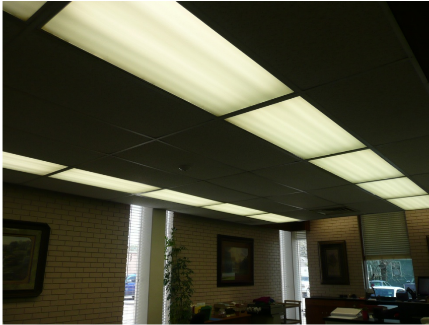
Figure 20: New Efficient T-8 Fluorescent Lamps (Utility Office)
