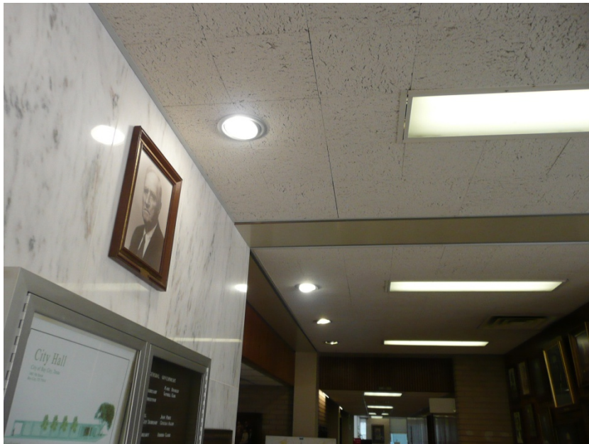
Figure 19: New Efficient T-8 Fluorescent Lamps (Main Lobby)
