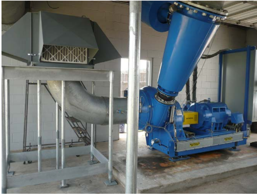
Figure 5: New 350 HP Siemens Turblex Blower
