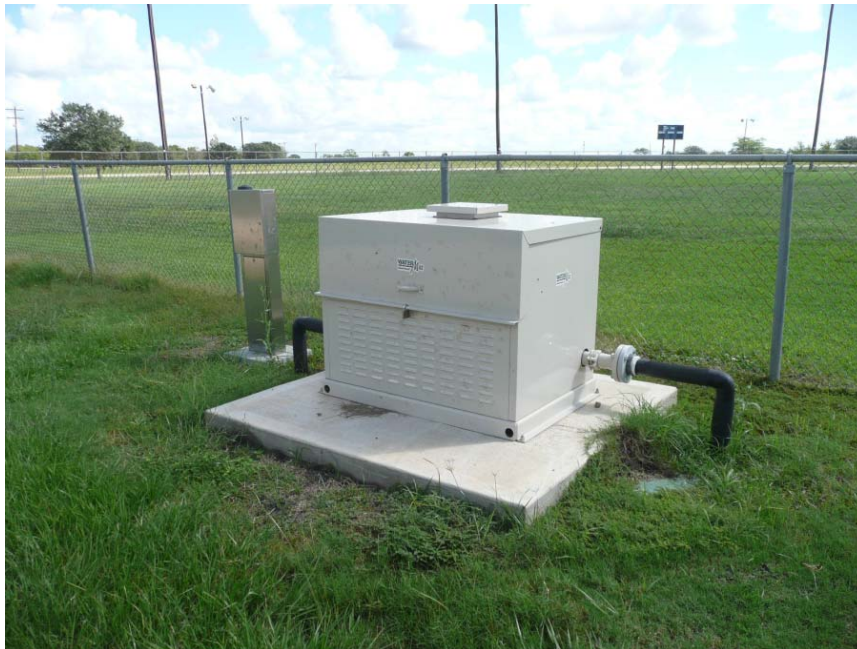
Figure 33: New Centralized Weather-Based Web-Enabled Smart Controller
