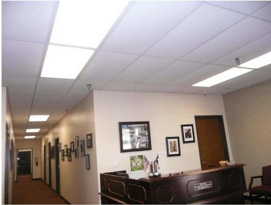
Figure 24: New Efficient T-8 Fluorescent Lamps (Chamber of Commerce & Ag Office)
