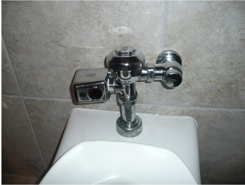
Figure 28: New 1.6 gpf Tank Toilet (Ladies Restroom); Auto Flush Sensor Was Observed
