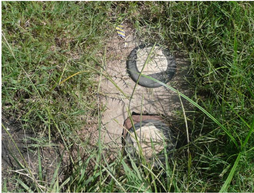
Figure 2: 2" Compound Water Meters
