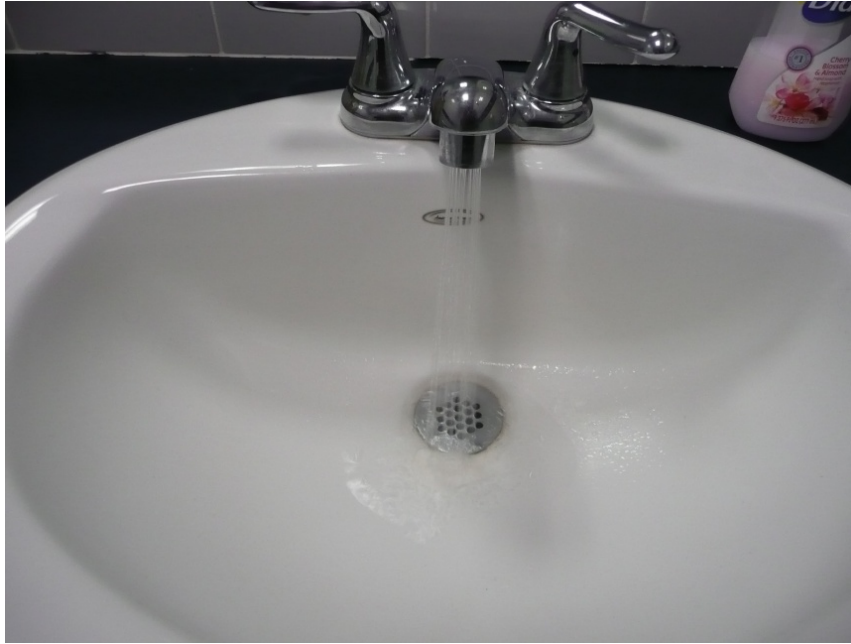
Figure 26: New 0.5 gpm Low Flow Aerator on Faucet (Ladies Restroom)
