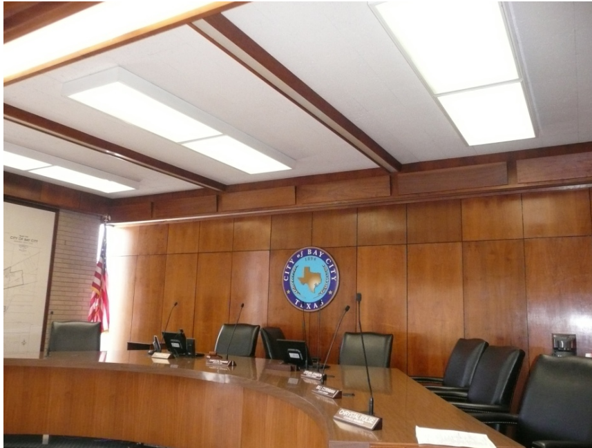
Figure 22: New Efficient T-8 Fluorescent Lamps (Council Chambers Alternate View)
