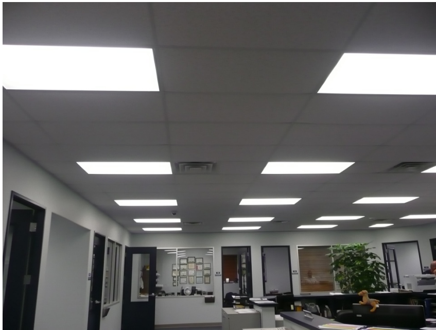
Figure 17: New Efficient T-8 Fluorescent Lamps (Main Office Alternate View)
