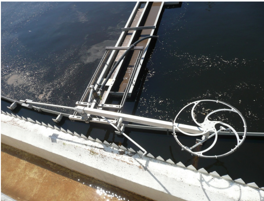
Figure 15: New Weir Cleaner
