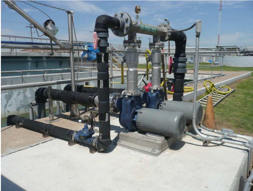
Figure 14: Two New 15 HP Non-Potable Water Pumps with VFDs (Alternate View)
