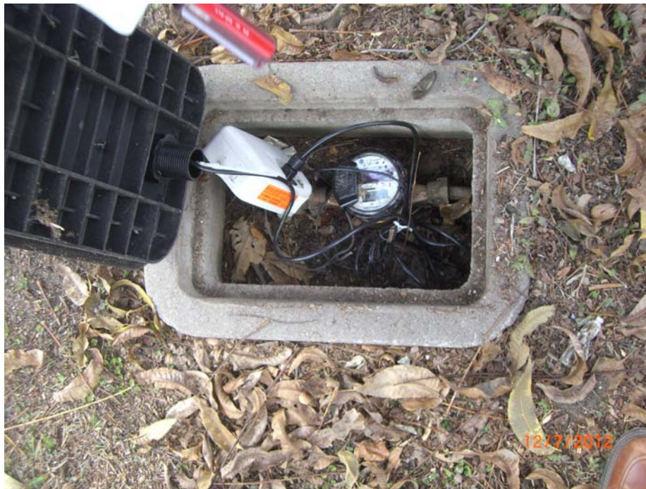
Figure 3: Radio Transmitter Attached to a Water Meter
