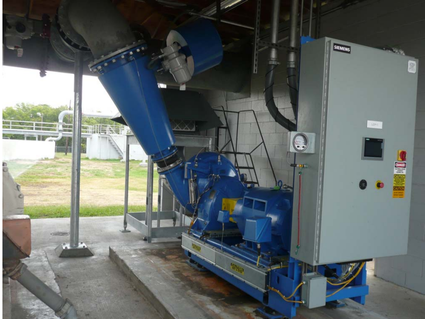
Figure 7: New 350 HP Siemens Turblex Blower (Alternate View)
