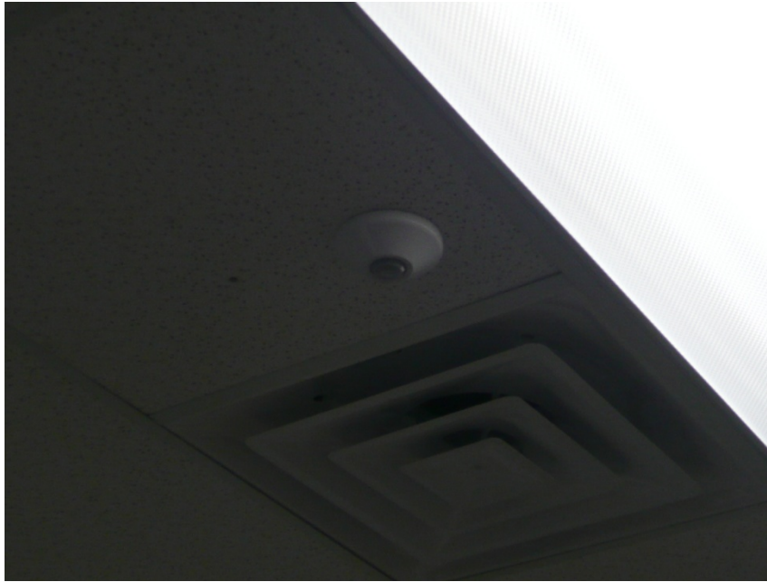
Figure 18: New Dual Technology Occupancy Sensor Lamps (Office)
