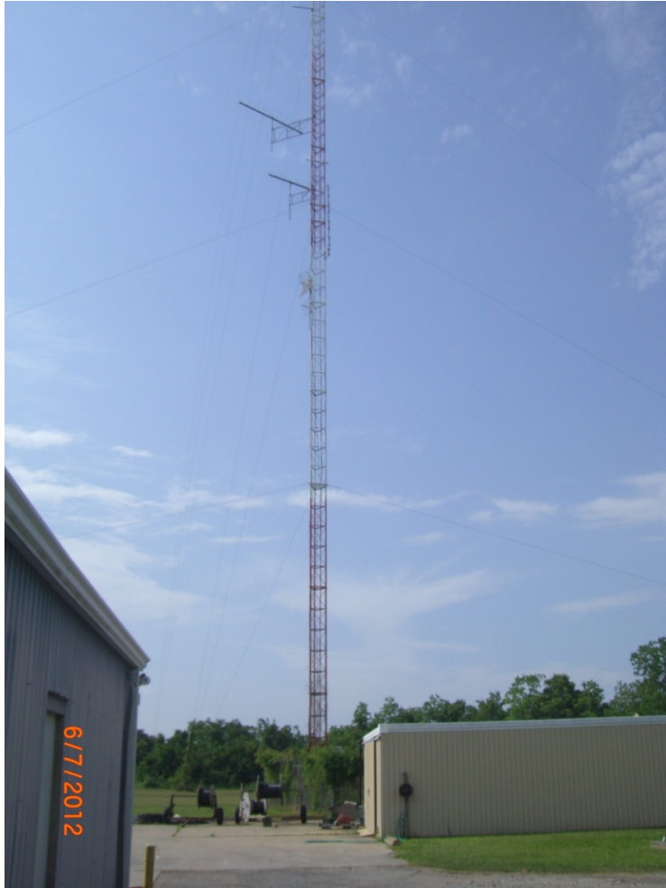
Figure 4: Fixed Base Data Collection Unit Installed on SCADA Tower at the WWTP
