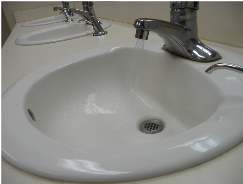
Figure 31: New 0.5 gpm Low Flow Aerator on Faucet (Ladies Restroom Alternate View)
