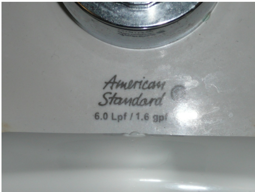
Figure 27: New 1.6 gpf Tank Toilet (Ladies Restroom)
