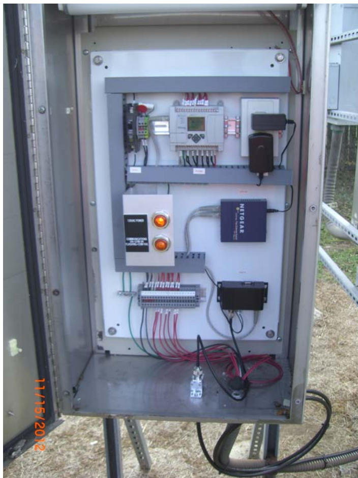
Figure 16: SCADA System Control Panel
