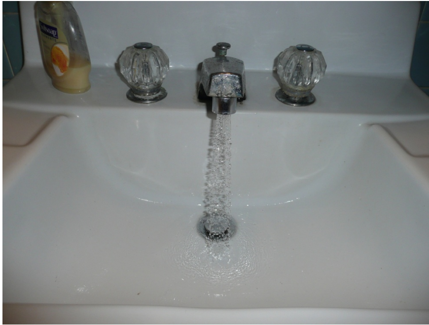
Figure 30: New 0.5 gpm Low Flow Aerator on Faucet (Handicap Restroom)
