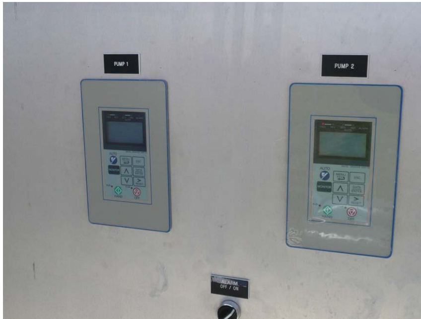
Figure 12: VFD Control Panel for Two Non-Potable Water Pumps
